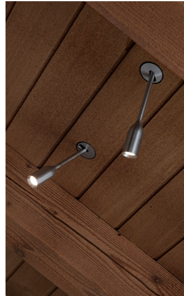
Project: Private Residence | Lighting design: ONE A
